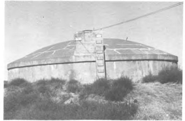
NORTH HILL HIGH LEVEL RESERVOIR
