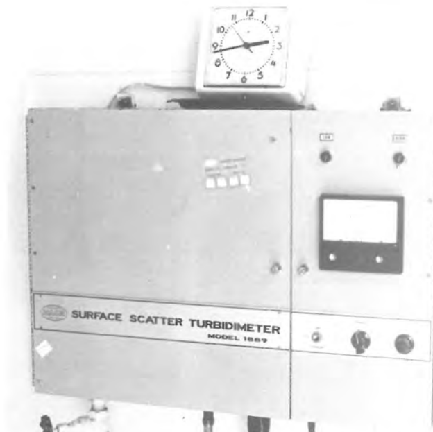
TURBIDIMETER IN WEIR HOUSE
