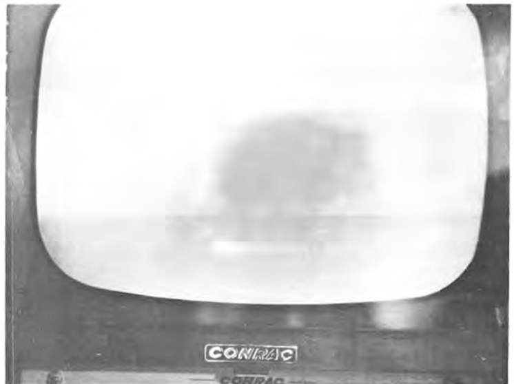
VIEW OF TELEVISION MONITOR SHOWING 12-INCH SEWER ALONG S.W. EMIGRANT AVENUE BETWEEN S.W. 6TH & S.W. 7TH STREETS. SEWER WAS FLOWING \frac{1}{3} FULL AND HAD NOT BEEN CLEANED. OBJECT ON LEFT OF PIPE IS SIDE SEWER STUBBED INTO MAIN.
