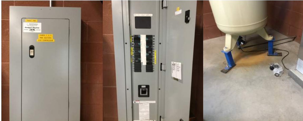
439 MBR Building Power Panel
