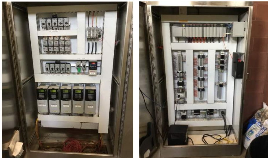
712 Primary Digester Complex Control Panel
