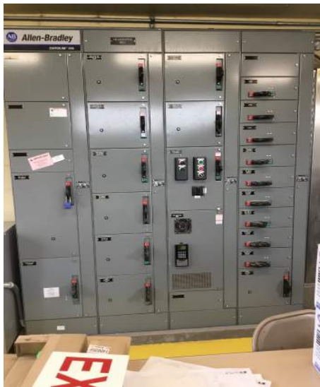
207 Headworks Motor Control Center
