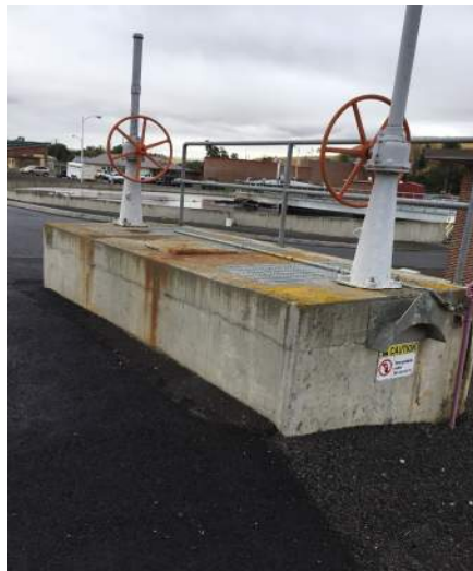
460 Secondary Control Junction Box
