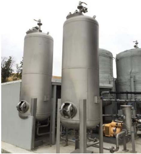
850 Cogeneration - Siloxane Removal system
