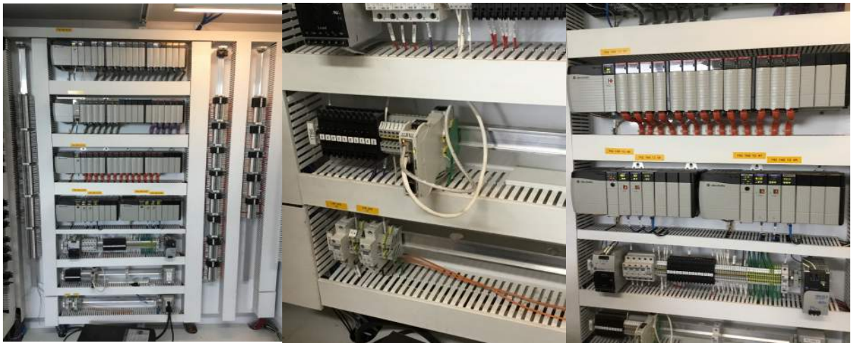
415 Secondary Process Building Control Panel
