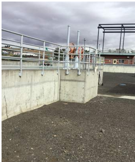
621 Chlorine Contact Chamber Splitter Box
