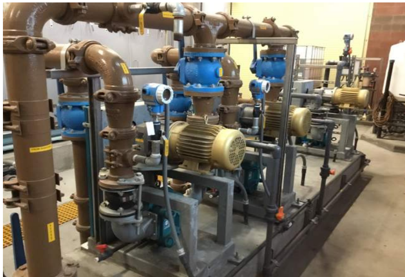
787 Dewatering Press Feed Pumps
