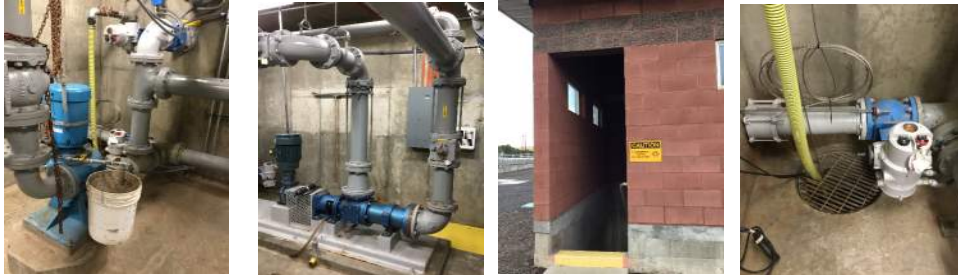
490 Underground Pump Station (WAS)
