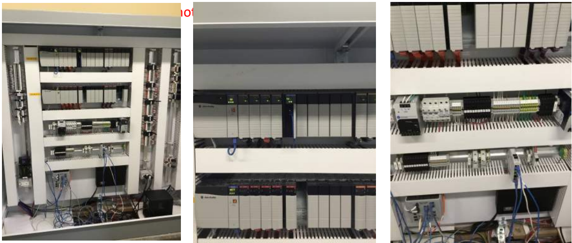
732 Solids Electrical Building Control Panel
