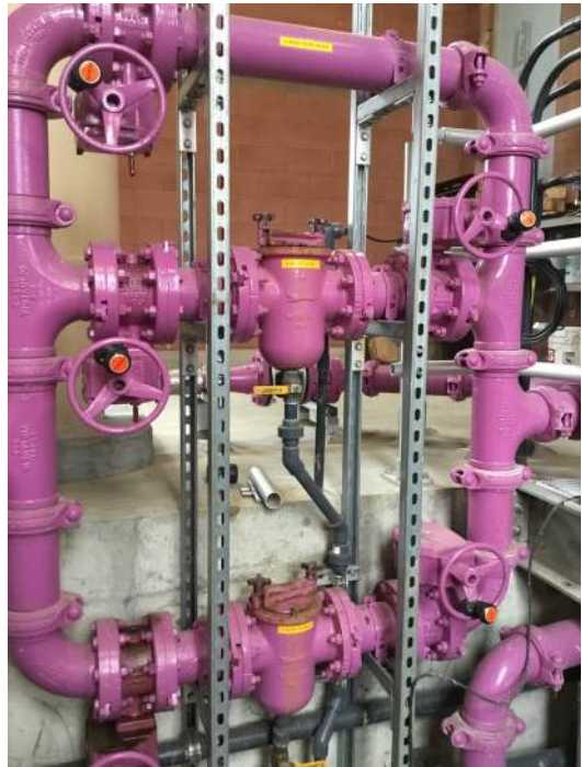
833 Utility Water System Filter
