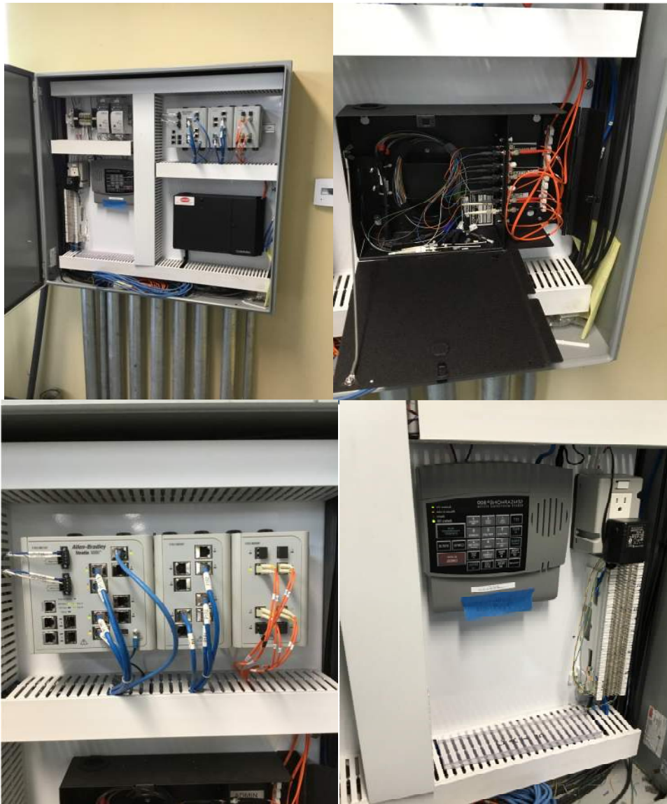
416 Secondary Process Building SCADA Alarm Panel
