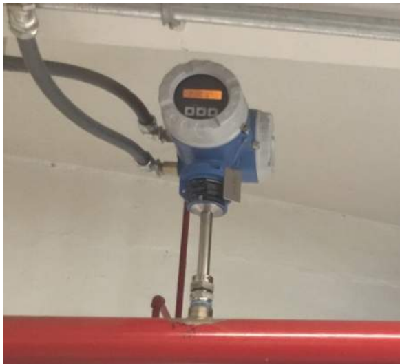
767 Secondary Digester Gas Flow Meter
