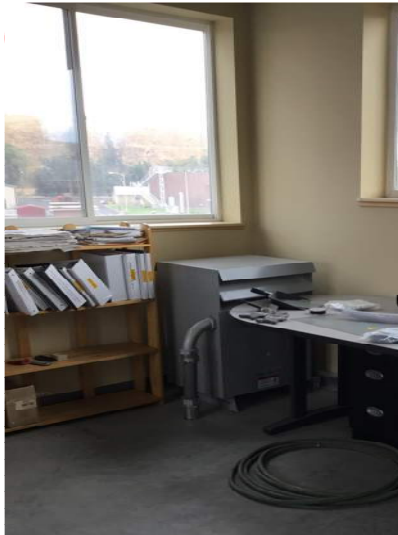
413 Secondary Process Building Dry Transformer
