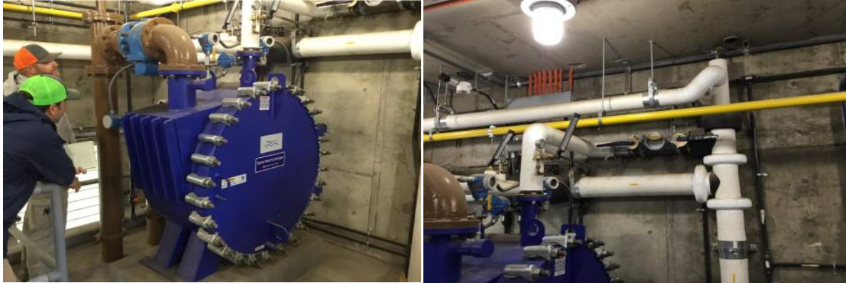
708 Primary Digester Heat Exchanger
