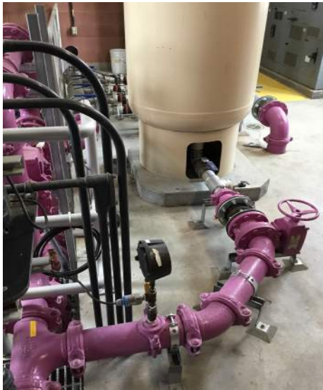
832 Utility Water Bladder Tank
