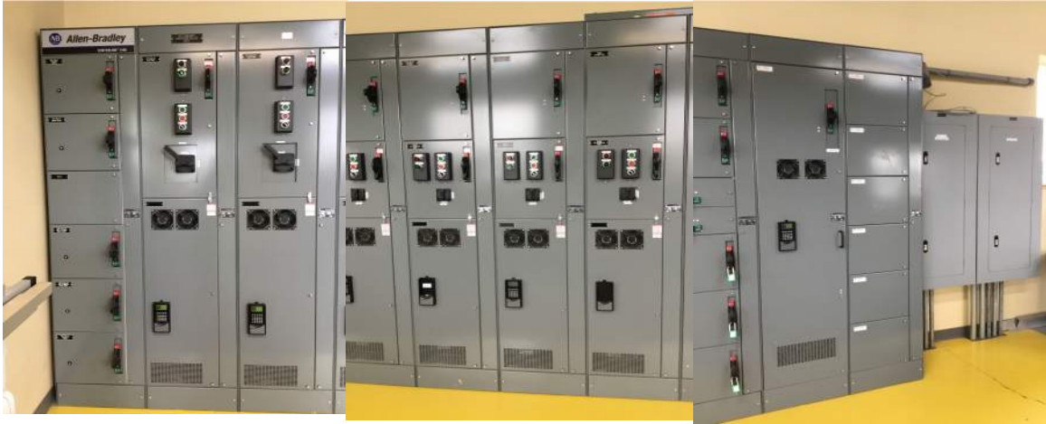
414 Secondary Process Building MCC
