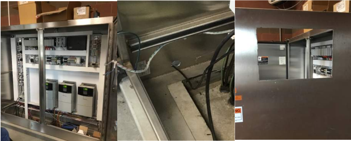
438 MBR VFD Control Panel
