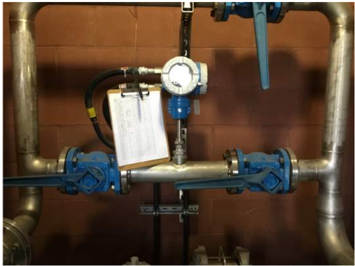
743 Gas Flow Meter
