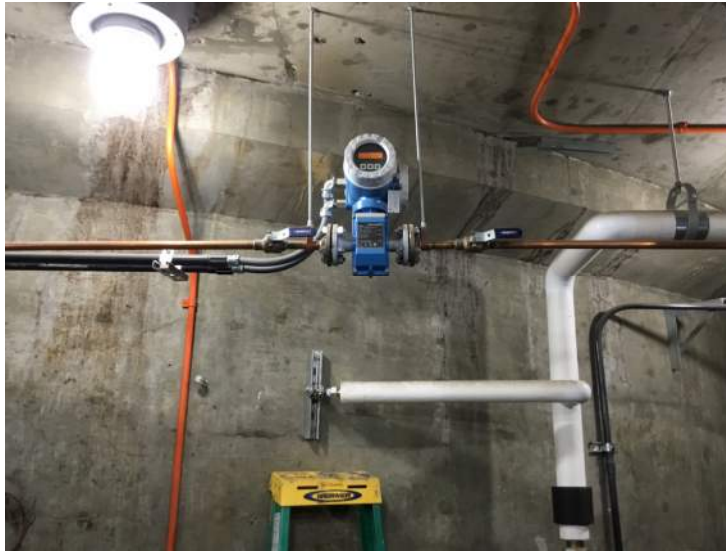
813 Boiler Gas Meter
