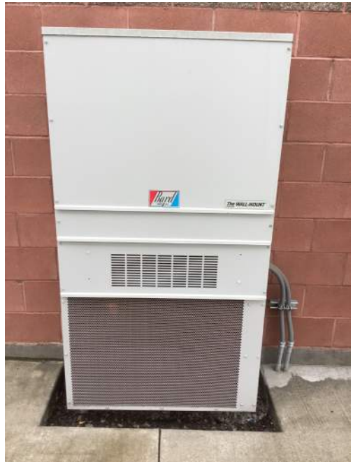
731 Solids Electrical Building HVAC
