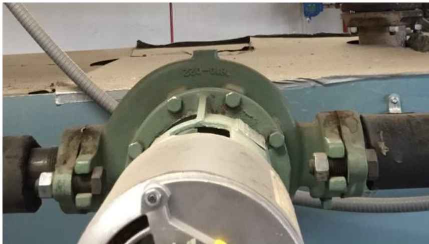
765 Secondary Digester Boiler Water Pump
