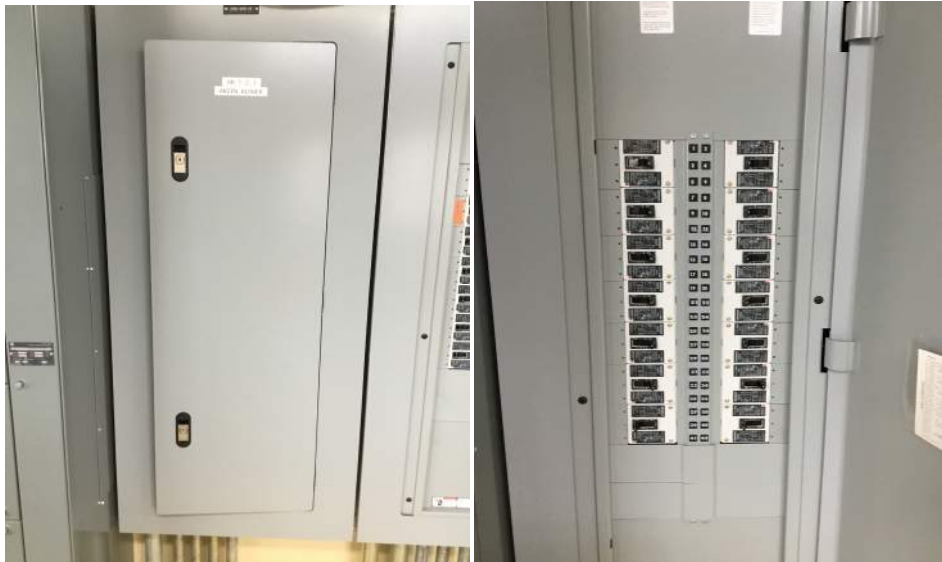
418 Secondary Process Building Aeration Flow Control Power Panel
