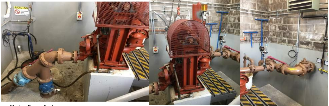
720 Primary Sludge Pump East
