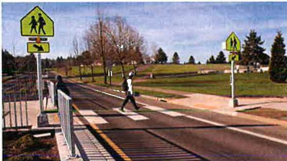
Rapid rectangular flashing beacon
