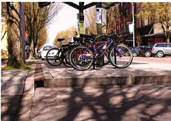
Slotted drain at retrofit curb extension
