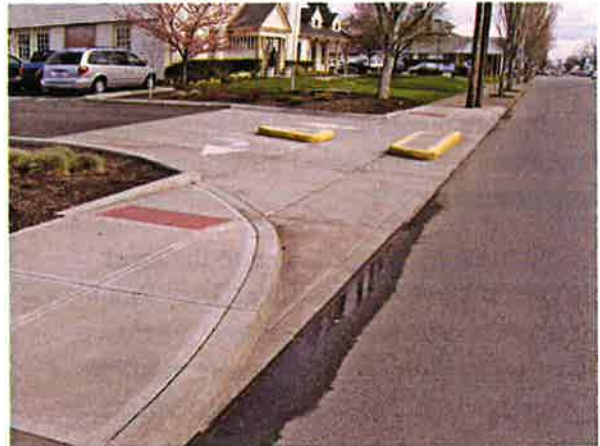
Commercial right-in, right-out driveway. NOTE: truncated domes are used ONLY at commercial style driveways.
