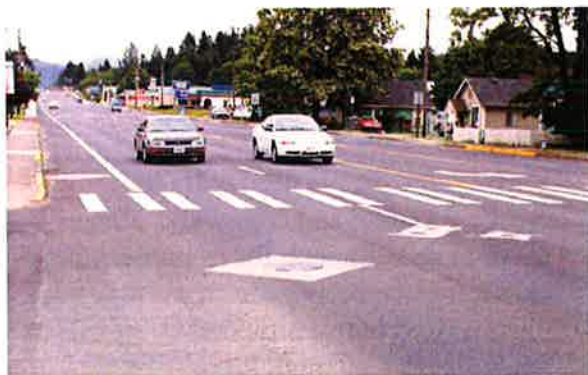
Staggering markings place stripes out of wheel paths
