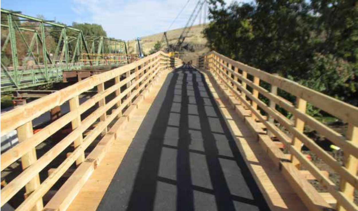
▲ The temporary work bridge included a pedestrian walkway to maintain residents' ability to cross the river during construction.
